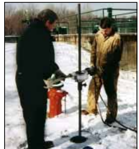
RS-2 operating a non-rising stem valve. An extension handle for two man operation is included with the machine.
